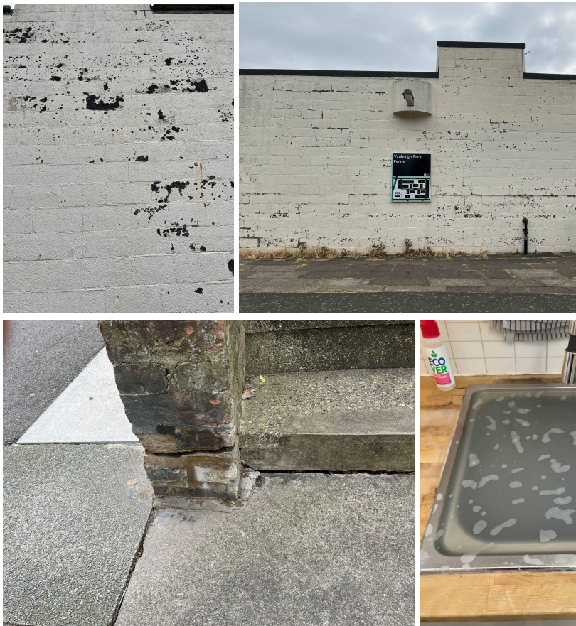
Above: Combe Mews showing deterioration of walls, subsidence effect on stairs, and overflowing sink due to blocked plumbing.
