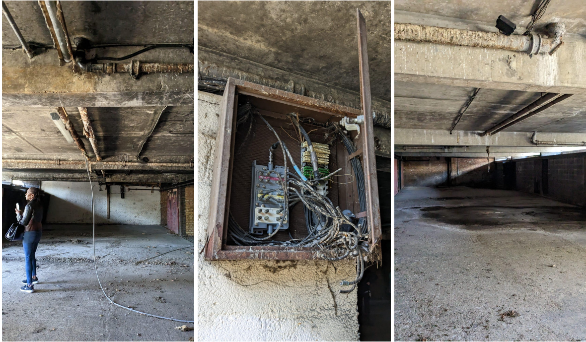
Above: the Undercroft beneath Combe Mews. Multiple health hazards from vermin, leaks, structural and electrical issues. Pigeon nesting in an open coaxial cable box. Leak below flat 3.
