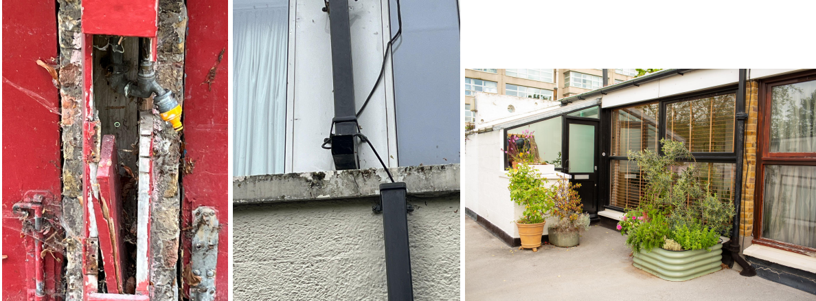
Above: Broken plumbing and guttering on Combe Avenue mews flats. Outdoor space used for small front garden with clear route to front door.
