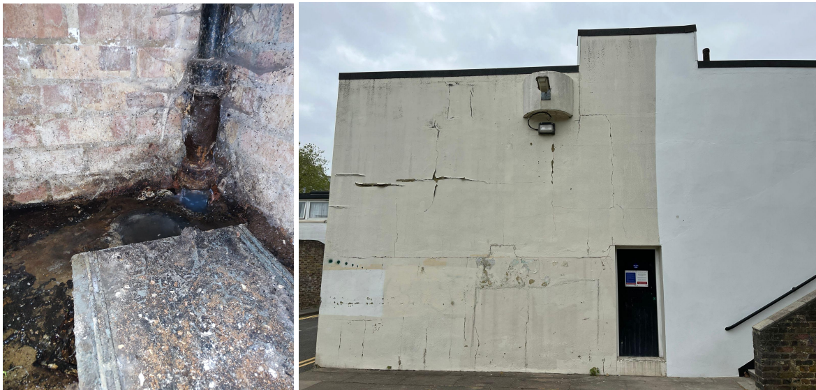
Above: images showing overflowing drain beneath Vanbrugh Park Road mews flats and superficial and partly finished wall repairs.
